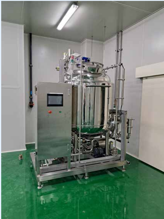
成品桶 Finished Product Tank
