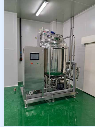
成品桶 Finished Product Tank
