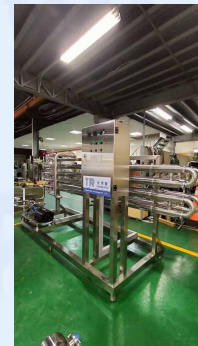
冷卻設備 Cooling Equipment
